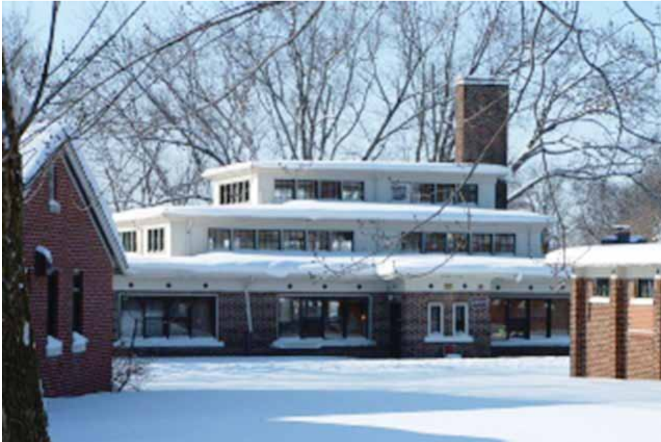
Lack of heating in winter accelerates deterioration
