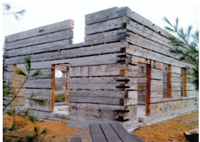
Petch House being reassembled at a permanent location in 2012, where it will be re-clad in traditional materials
